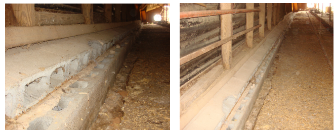
Figure 14. No vertical steel in concrete block side wall.
