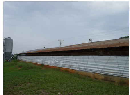
Figure 27. Poultry house with possible truss damage.
