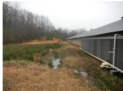
Figure 7. Standing water can lead to foundation problems.
