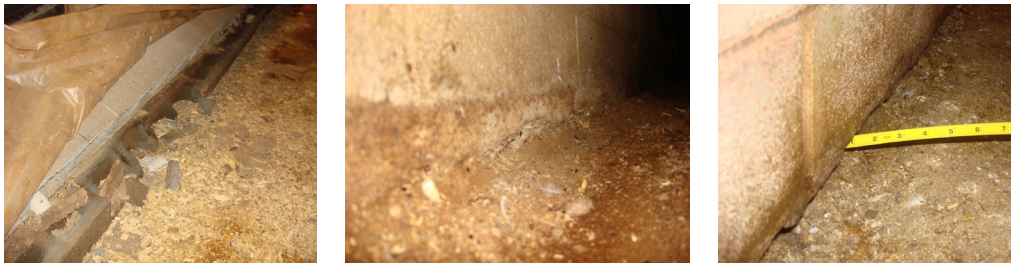
Figure 20. Erosion of block caused by manure.
