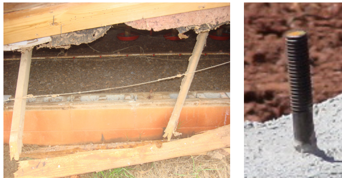
Figure 16. Cores of block should be filled intermittently and J-bolts installed to connect plates to the foundation.
